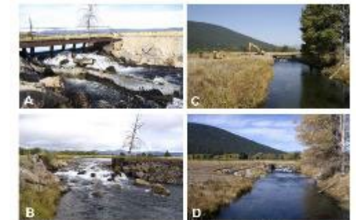
Figure 9-16: Photos of the work site showing the main channel diversion before construction (A) and to allow its replacement with a rock weir during the project (B), as well as showing the entire main channel before construction (C) and following replacement of diversion structure, channel roughening, and the addition of a fish bypass on the left following construction (D). Photos reproduced with permission from Trout Unlimited.
